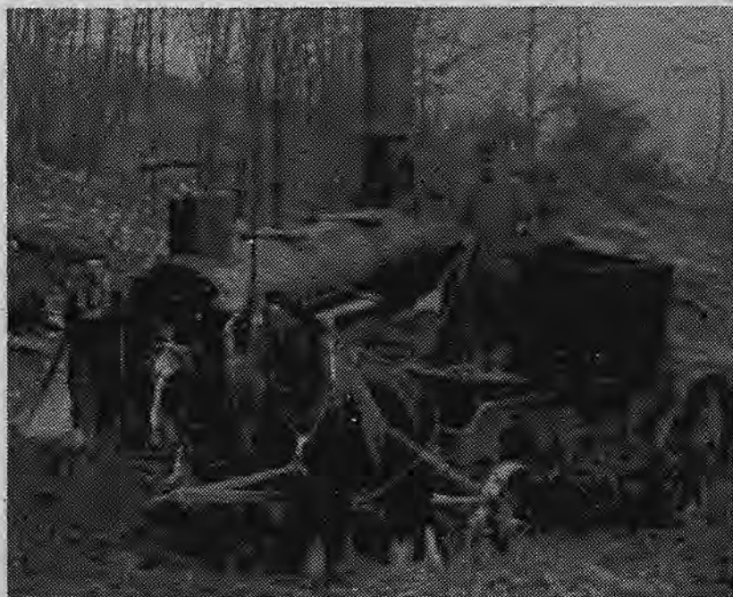
Building the first Warwick-Greenwood Lake State road in 1913. Henry Babcock, Sr. with team.
